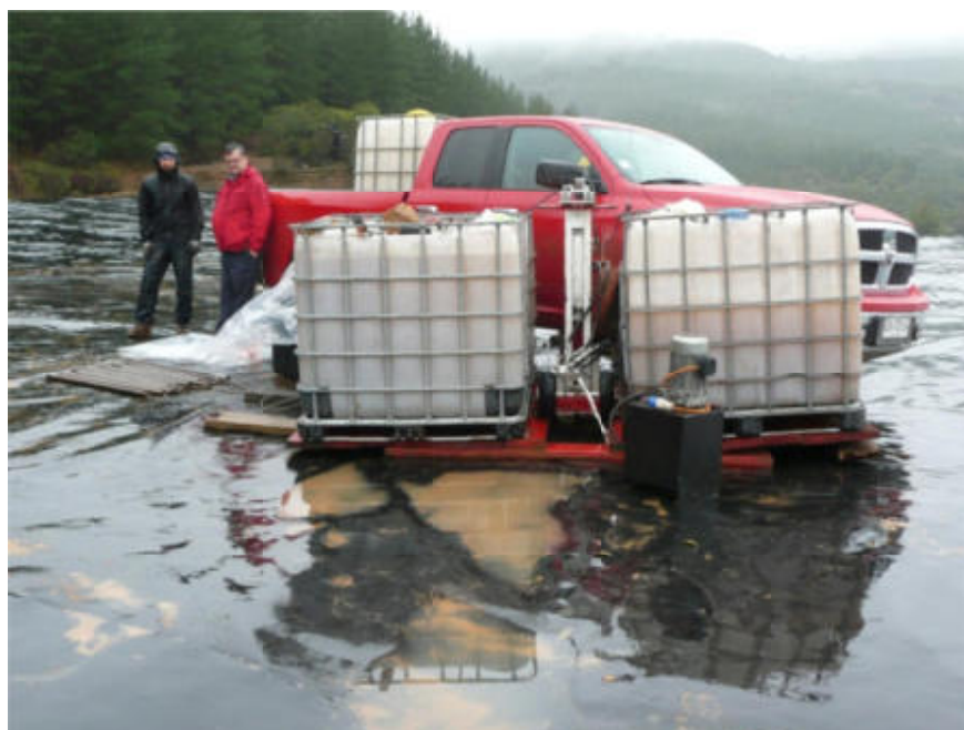
Figure 5.1 Portable “ramset” mobilized for Las Palmas field investigations because of the difficult access conditions. The reaction weight was provided by water tanks and truck. The ramset is the white hydraulic jack in the middle. The black box with orange cord to the right is the hydraulic pump.
